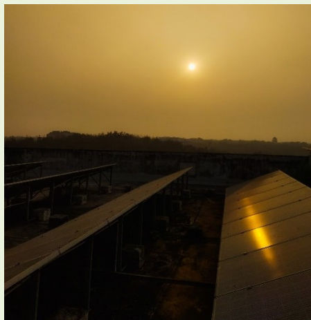
Fig. 4: Use of solar power panels in TU Campus
